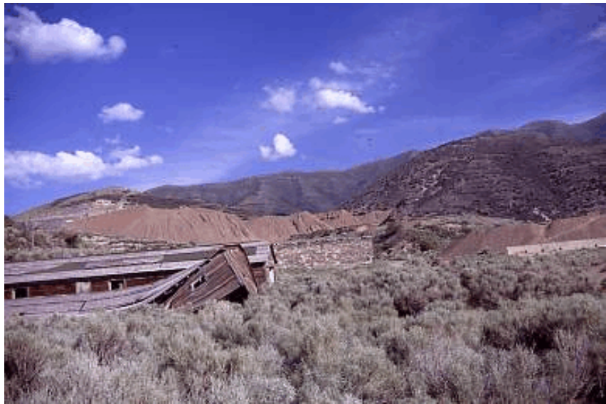
Another view, building falling down, overburden of the vein in the background.
